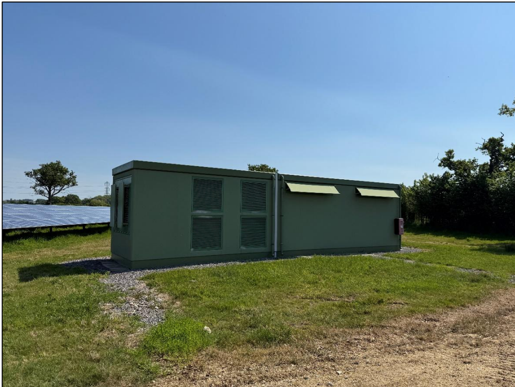
Image 4-56 Typical Conversion Unit / 33kV Sub-distribution Switch Room.
