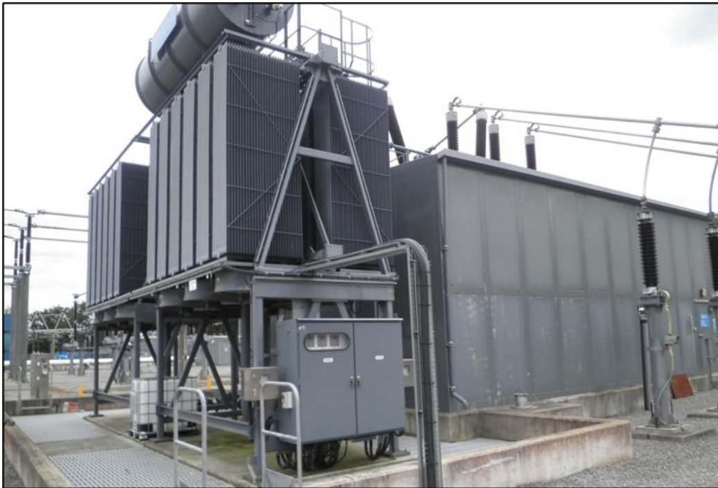
Image 4-67 Air insulated Substation
